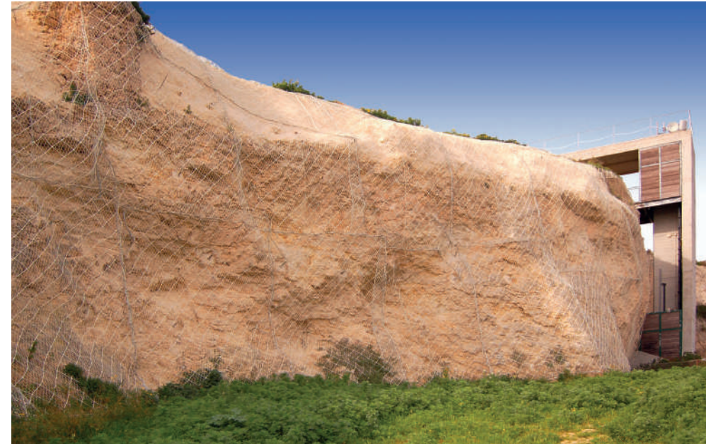
Municipality of Cagliari Consolidation and safety of the rocky ridges of Colle di San Michele. Deep nailing with Gewi threadbars diam. 40mm on structural scaffolding and installation of coloured steel mesh.
