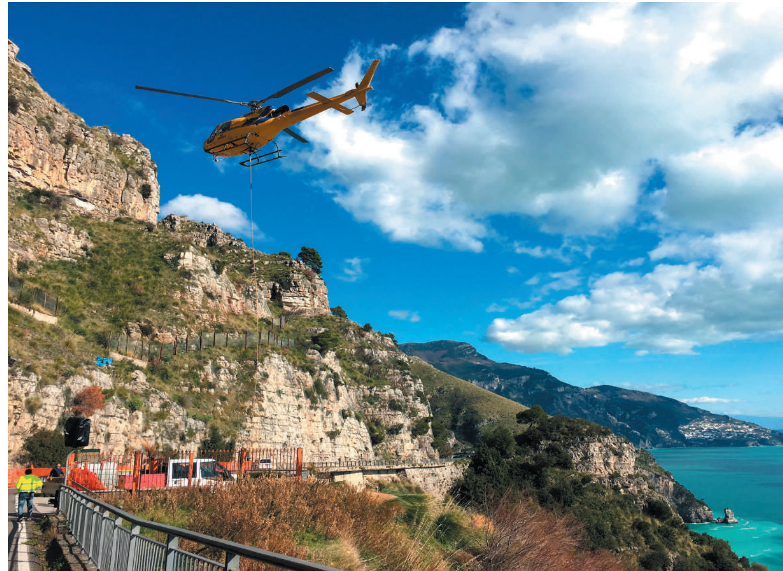
▼ SS 163 Amalfitana Installation of rockfall barriers and wire mesh by use of helicopter.
